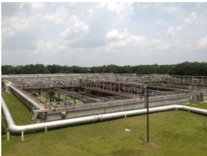
Some of the plants many aeration basins.
