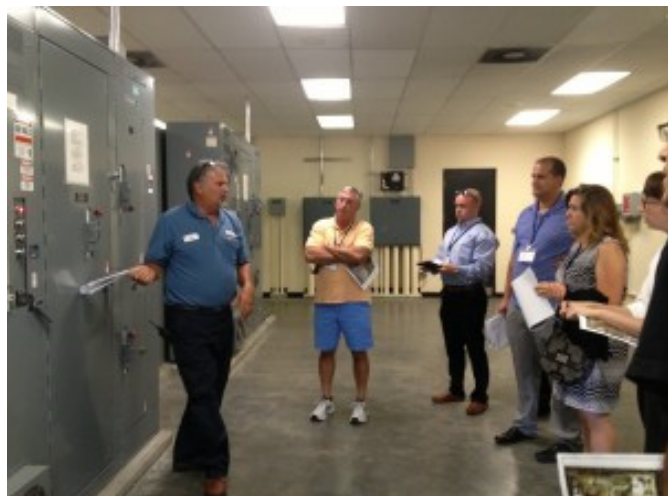
Tom shows us the plant's new VFDs for the raw lift pumps
