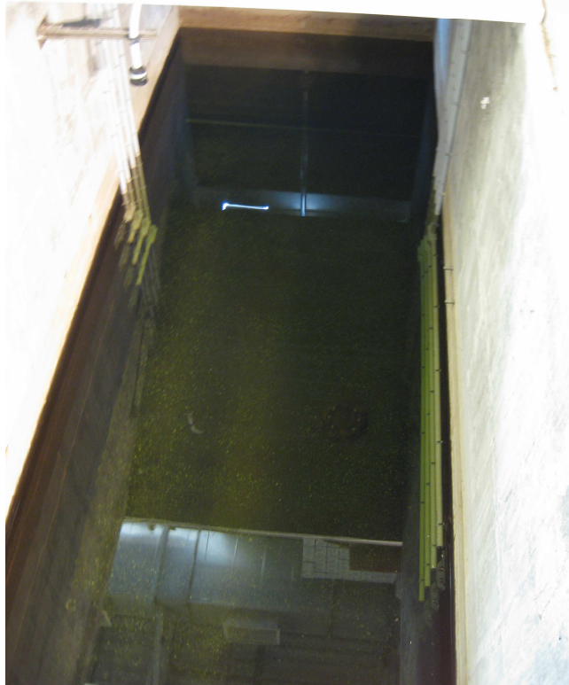
Photo 2. UV - Open Channel Multiple Path Transit-Time Flowmeter Installation
