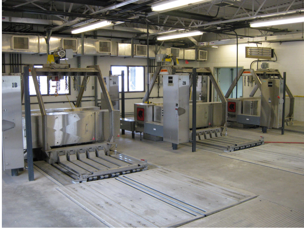
Photo 3. UV Installation at Clark County Water Reclamation District
