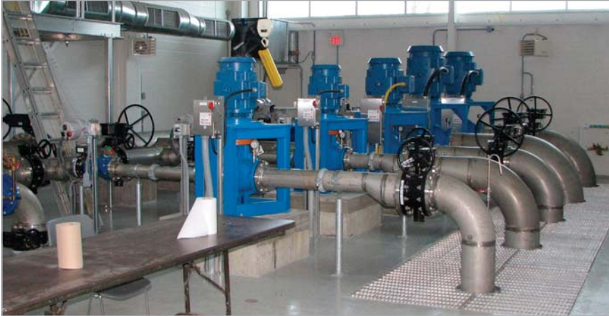
The City of Guelph's Clair Road pumping station was used as a pilot project to test a new PLC platform as part of its SCADA Master Plan.
