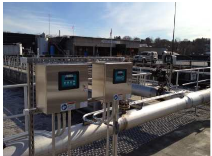
New DO instrumentation and valves for the aeration basins.
