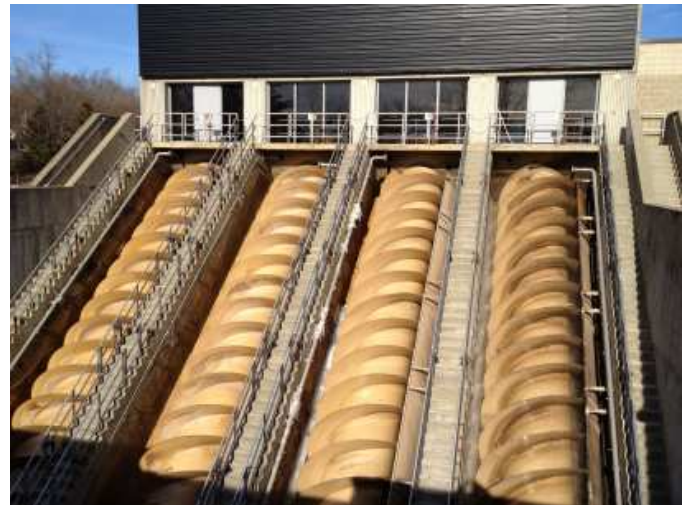
New Influent Screw pumps installed at the plant headworks.
