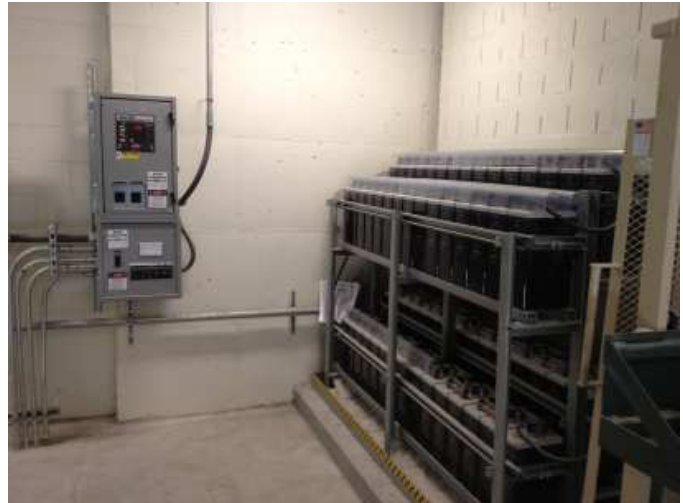
Battery room for the new plant-wide centralized UPS System.
