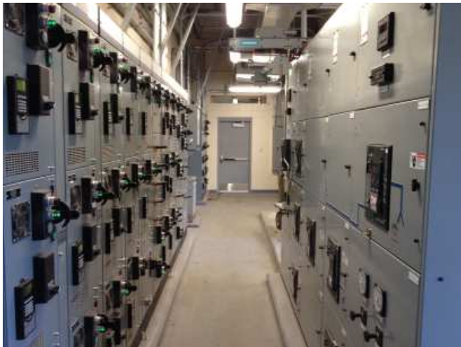
New Electrical Room and MCC equipment
