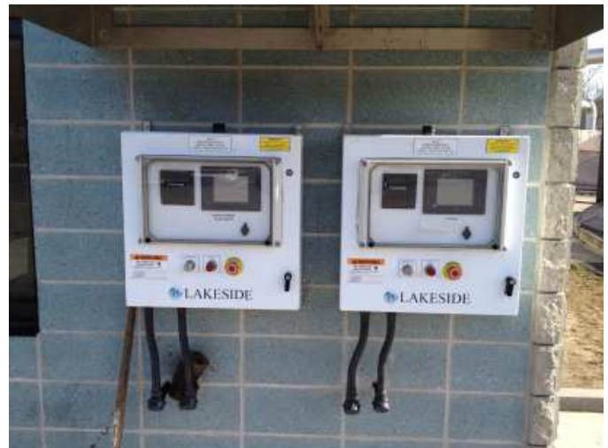
New Hauled Waste System Operator Terminals in the septage receiving area. Notice the large Emergency Stop buttons for the loading pumps.
